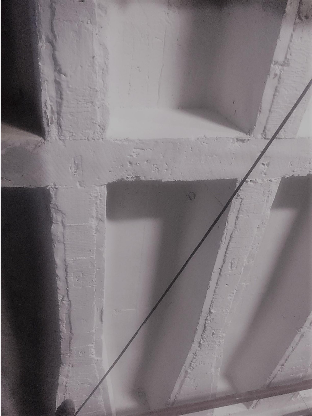
Below: The underside of a heritage waffle slab, applied with intumescent paint
